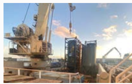
Mobilisation of concrete silo for a grouting operation at an offshore wind farm
